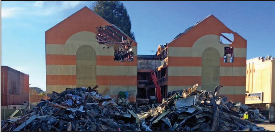
Demolition of Oxford Court (Muller & Caulfield, architects, c. 1983) in November 2021. Anthony Bruce
