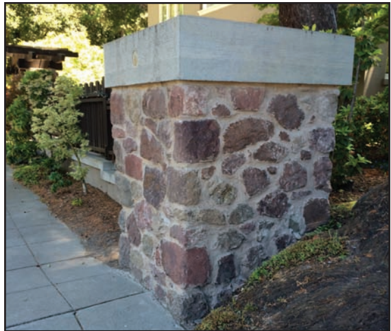
Newly built pillar at the northeast corner of Claremont Avenue and Hillcrest Road, and the offending root base, which has spread out onto the sidewalk. Anthony Bruce, 2017.
