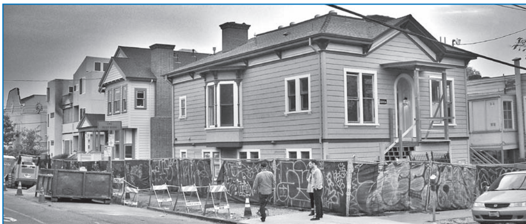
The Woolley House (1876) under renovation, after re-siting at the corner of Regent Street and Dwight Way. At its left, the Blood House (1891); the Needham-Obata Building (1907) is at the left edge. John McBride, 2015.
