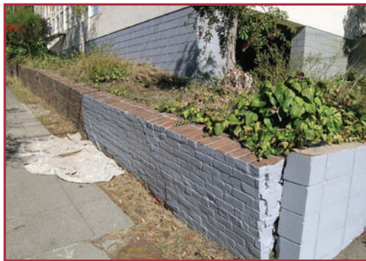
The clinkerbrick retaining wall on La Loma Avenue in the process of being painted. Daniella Thompson, 2008.
