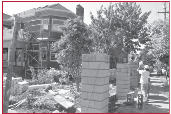
The Lacey House with its exterior readied for stucco and the concrete block wall under construction. Daniella Thompson, June 2006.
