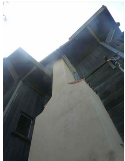
(Above, upper exterior wall and roof detail of north elevation of main house. Note the wide eaves, brackets, board and batten on upper floor, horizontal board siding on main floor, and wooden “posts” expressed on the exterior. This is looking southwest, towards the upper portion of the second floor, with the stairwell bay at right. Photo S. Finacom, 2021)
