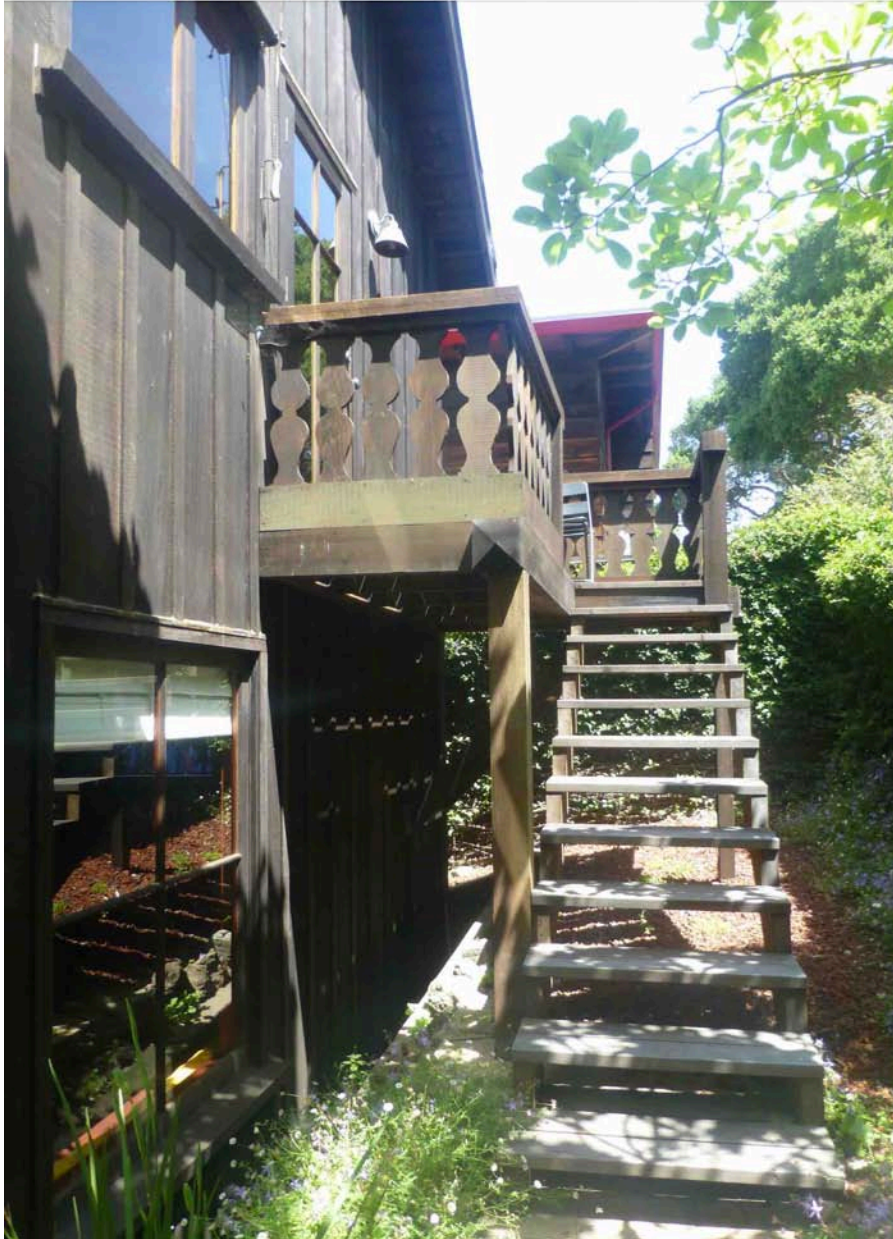
(At left, east end of addition showing balcony and staircase that altered the original “Juliet” balcony in this location. Kroeber study is lower left. Photo S. Finacom, 2021.)
